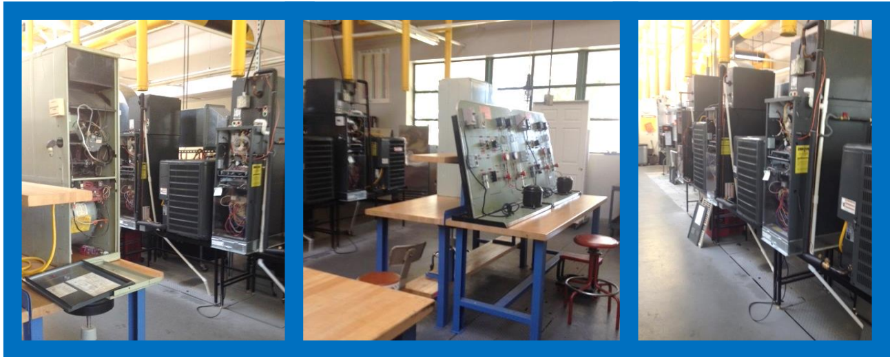
Air conditioning units and controls in Alan's teaching lab in the OE building.
